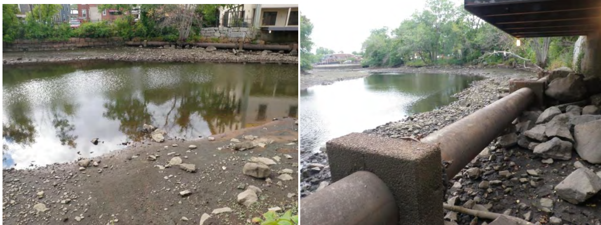
Exposed Sewer Force Main Crossing Beneath Choate Bridge River Left
