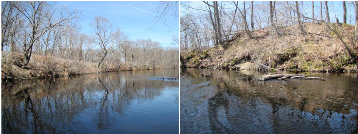
Railroad Embankment River Left Across from IRWA Office Far-field View (left) and Close-up (right)
