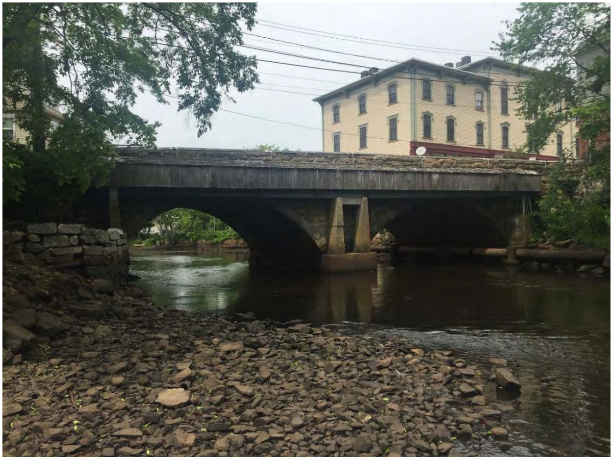
Figure 7. Looking upstream at Choate Bridge during low flow and low tide conditions
