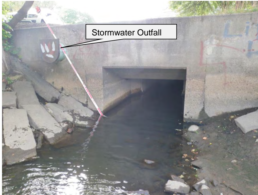
Farley Brook and Stormwater Outfall Entering River Beneath Parking Lot River Left
