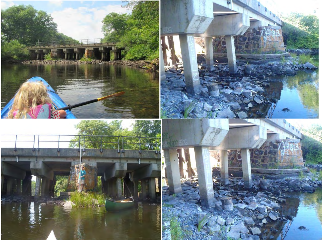
Railroad Bridge Views (Photos Taken During September 2016 Drawdown) from Upstream (top two rows) and Downstream (bottom two rows)
