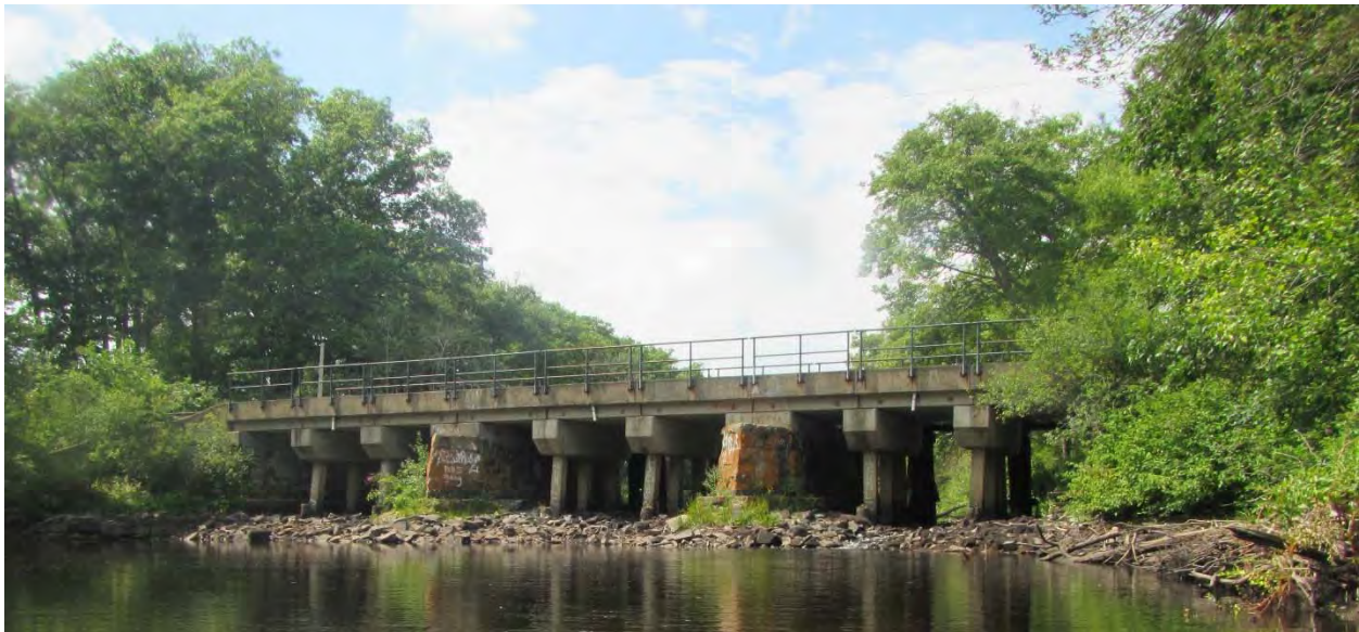
Figure 6. Looking upstream at the railroad bridge taken when the impoundment was drawn down showing accumulated rock on the bed (photo credit: Horsley Witten Group)
