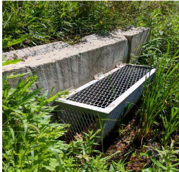
Shady Brook Culvert Downstream End (left), Shortly Downstream (right), and Upstream (bottom)
